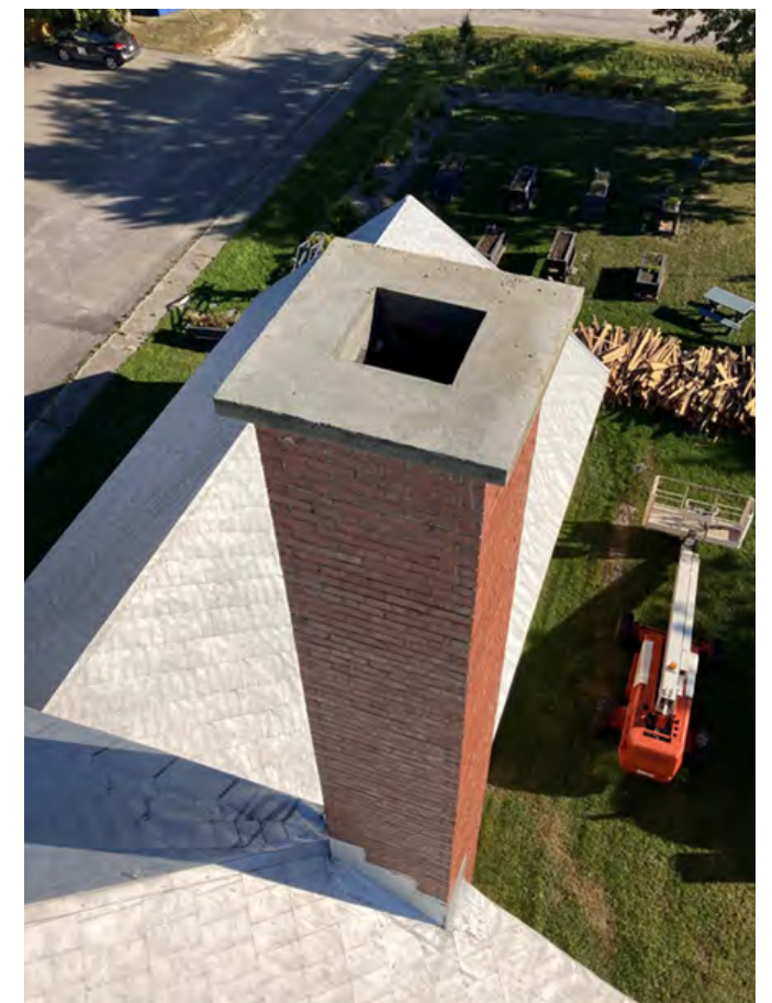
The newly renovated chimneys of the Saint-David de Sully church, in Quebec. Photos by Steve Thériault.
